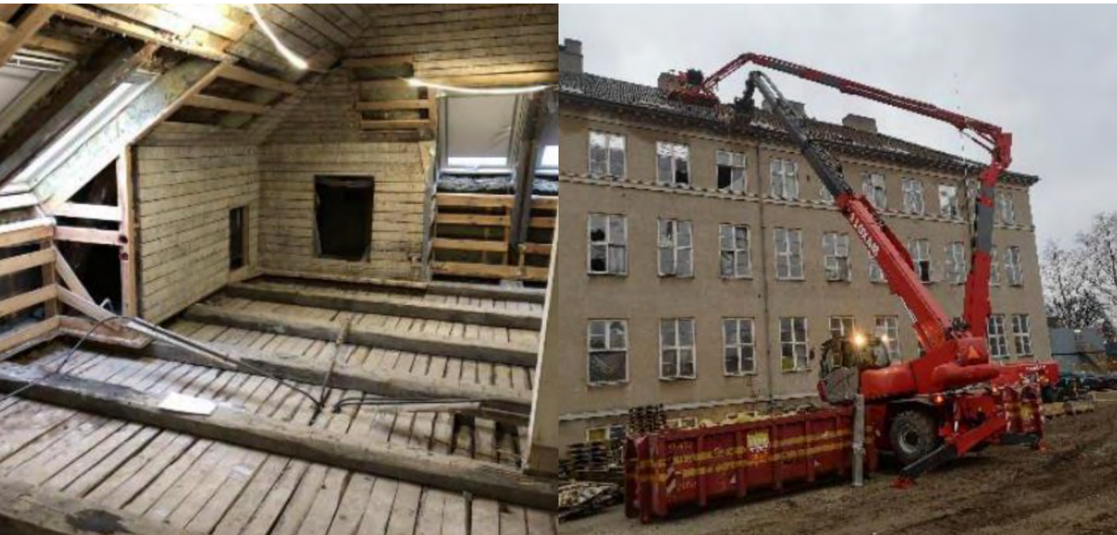
Selective demolition of buildings: The Rockefeller-Centre, The National Hospital, Copenhagen 2018-2021. The photo on the right shows dismantling of roof tiles for reuse. The photo on the left shows interior locations after stripping of loose items, insulation etc.
