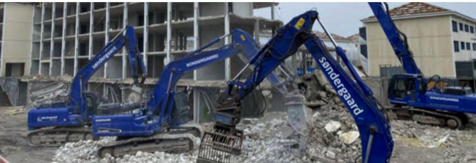
In Taastrupgård, a social housing building neighbourhood in Høje-Taastrup, the concrete from the demolished building has been crushed to serve as aggregate for the foundations of the New City Hall.
