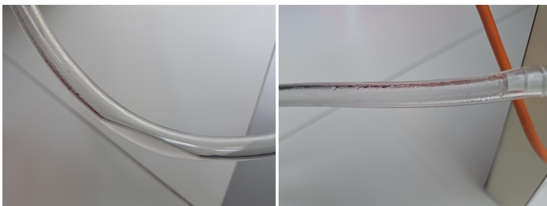
Figure 4.4: Images of Condensation forming in the exhaust tube and beginning to pool at a low point in the tubing, after exiting the SVC chamber. This indicates that the solvent has exceeded the saturation pressure.
