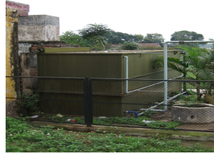
The new wastewater treatment plant at Phú Thọ Town General Hospital
