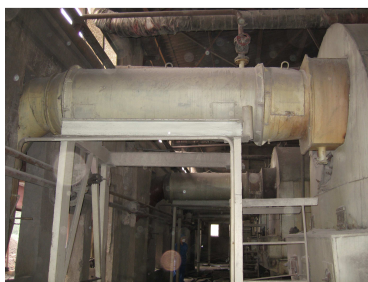
The one part of a boiler
