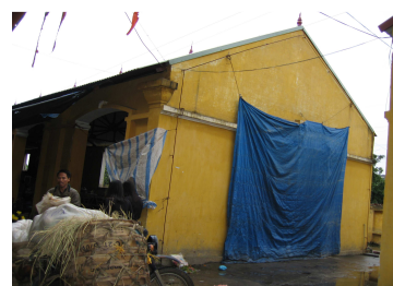
The side opening of the restaurant of Gát market is covered with nylon sheets when it rains.
