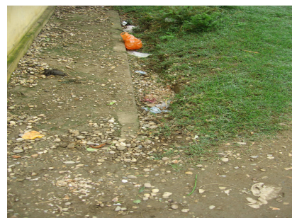
...whereas this end of the drainage system has no outlet
