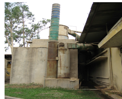
Part of the dust suction system
