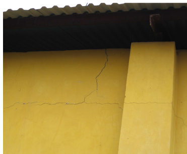
The walls are cracked on both sides of the restaurant...
