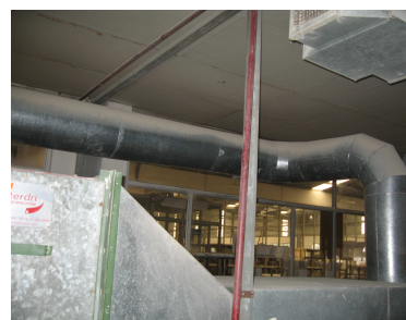
A part of the heat recovering system
