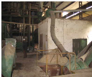
Part of the grinder
