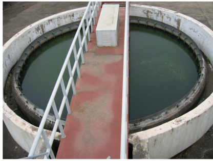
A part of the upgraded wastewater treatment plant at Phú Thọ Provincial General Hospital
