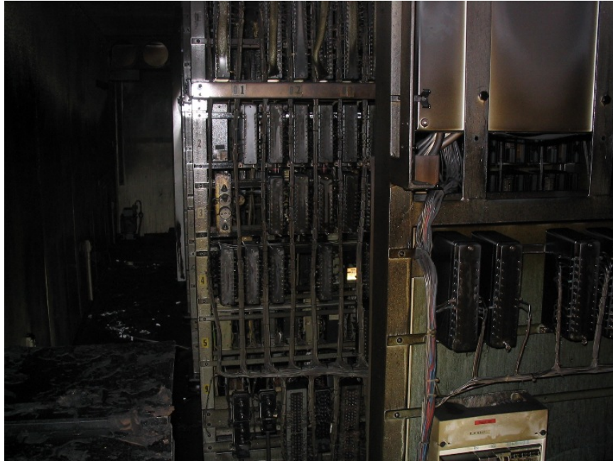
Figure 6.1: An explosion of a remote control room due to a short-circuit.
