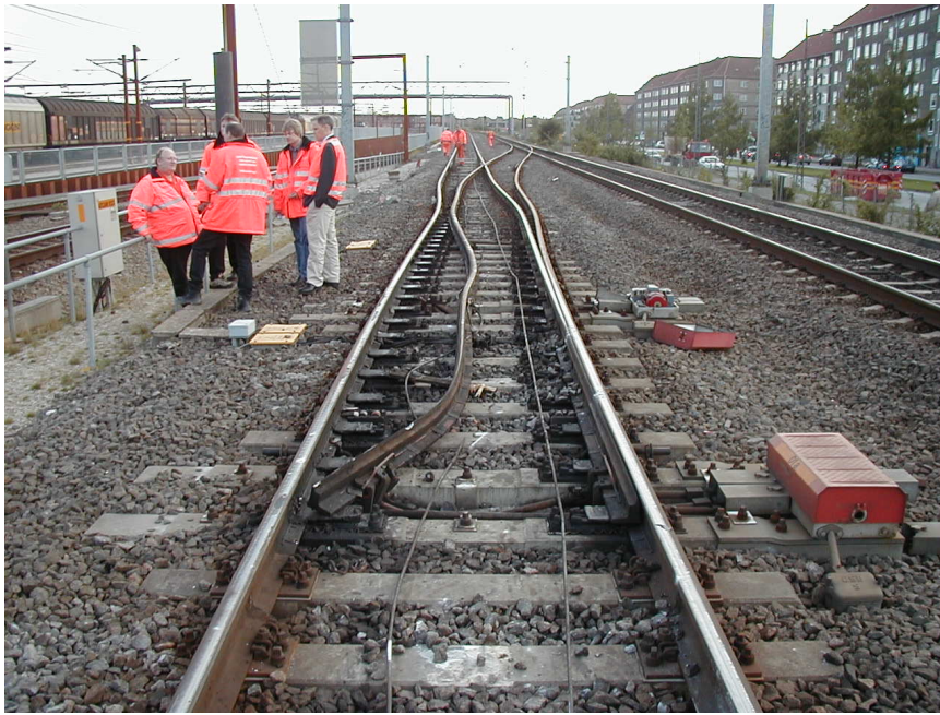
Figure 7.7: A damaged track switcher. The red box on the right side of the picture is the automatic box, that receives all signals from the control room user interface
